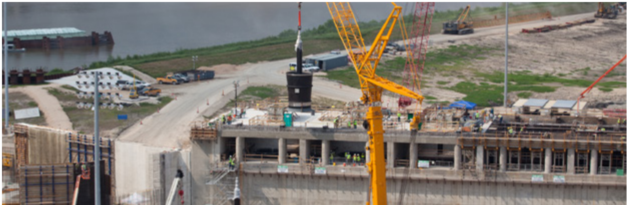
Photo: Pentair's massive pumps are installed at the Gulf Intracoastal Waterway in New Orleans.
