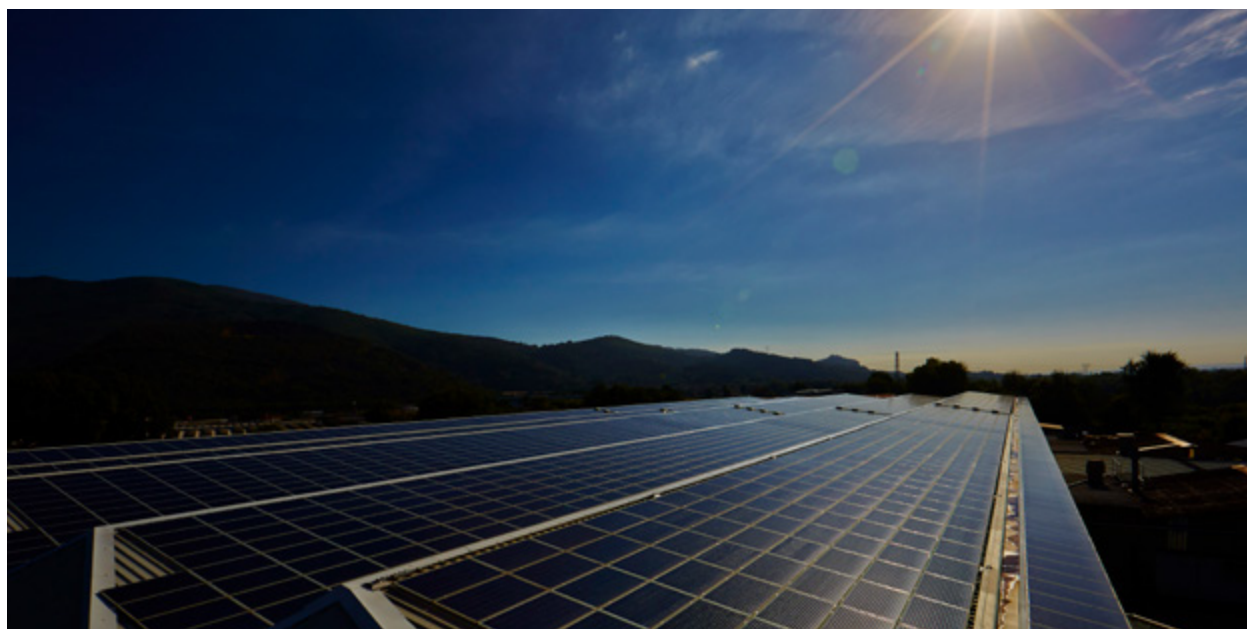
Photo: A solar roof on Pentair's manufacturing facility in Pisa, Italy.
